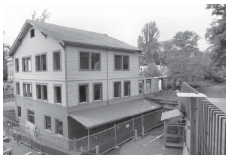
The south end of Johnson Annex gets a reprieve. The top two floors once held Atmospheric Science classrooms and offices.
